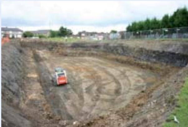
Stage 1: Calculate volume required and excavate site, allowing for 2m depth of burial
