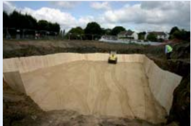
Stage 2: Protect the integrity of the root barrier membrane with a layer of sand and provide shutter ply supports for the edge of the cell.
